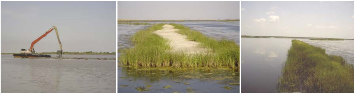
Figure 1.1. Terraces under construction (left), recently planted (center), and completely vegetated (right) at Sabine National Wildlife Refuge.
