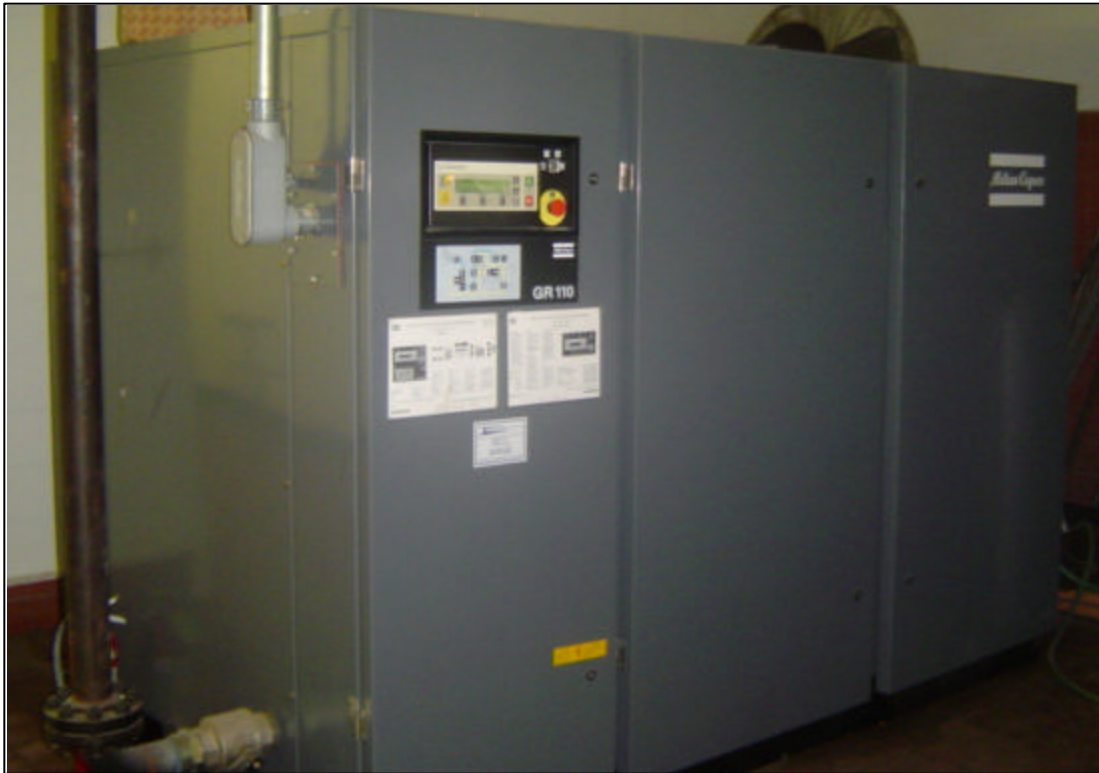
Figure 3.5 The high-pressure compressor
