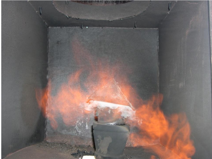
Photo C: Syngas being flared during gasification.
